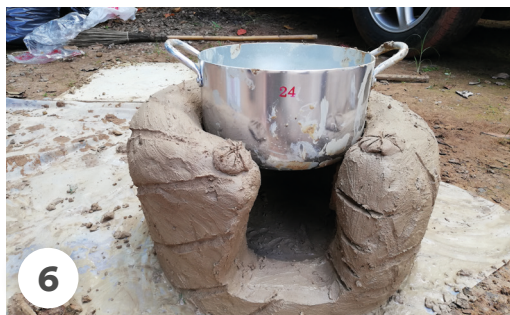
6 Leave to dry naturally. Once dry it can be carefully moved to another location if built on plastic.
