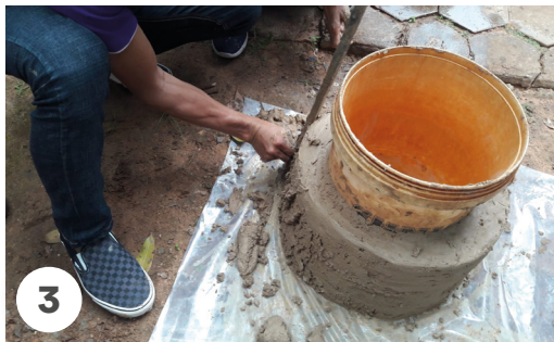
3 A small part of the three bricks are embedded in the wall (as in picture 5B) but the bigger part of the bricks are left on the inside of the walls to hold the pot. The walls should be around 4–5cm thick (see blueprint p. 27).
